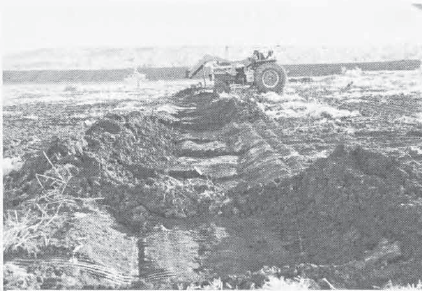
Plate 32 Gap spreader banks were constructed to safely spread runoff and prevent erosion of a sloping bare area on Hodgson River Station (12 January 1993).
