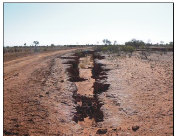
Photo 2: Erosion adjacent to a road within the Tennant Creek Pastoral District.
