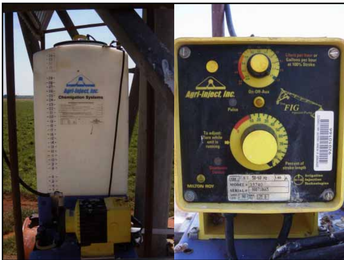
Figure 23. Chemigation unit used for applying pesticides through irrigation water
