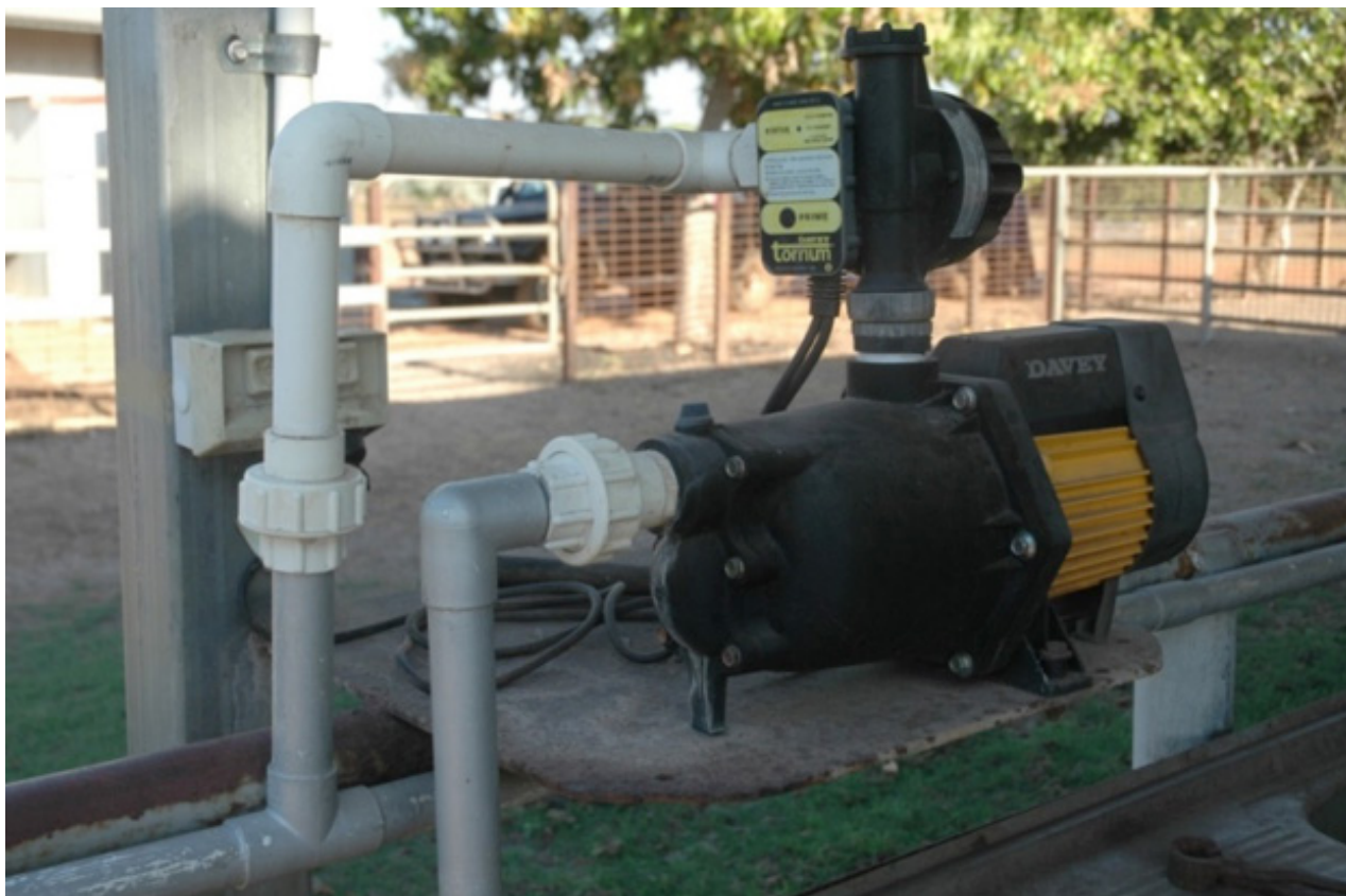
Figure 11.15 A simple pressure pump. This can supply water to troughs, washing facilities and run a sprinkler system for keeping dust levels down and buffalo cool. Small systems could use a 12 Volt pressure pump similar to those used in spray packs.
